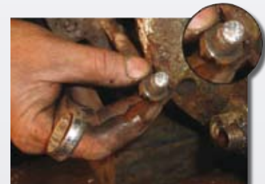
...which can lead to broken bolts.
